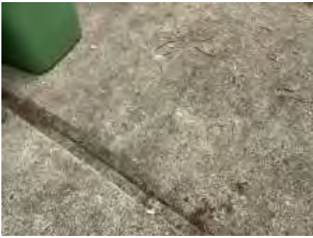
Settlement cracks to parts of the pathway/driveway. Recommend engaging a concreting contractor to repair/replace and avoid further deterioration
