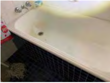
Cracked/loose/missing sealant/grout to parts of bathroom. Recommend resealing to reduce the risk of water leaks and damage
