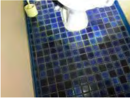
Cracked/loose/missing sealant/grout to parts of bathroom. Recommend resealing to reduce the risk of water leaks and damage
