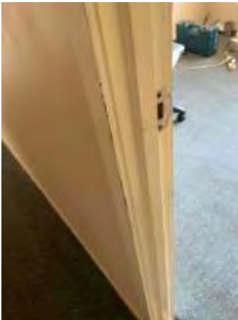
Showing example of scuff marks and paint blemishes
