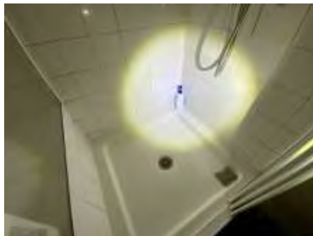
High moisture readings to the walls around the shower. Recommend engaging a builder/plumber for further inspection to determine if the shower needs re-building/waterproofing or it can be repaired easily
