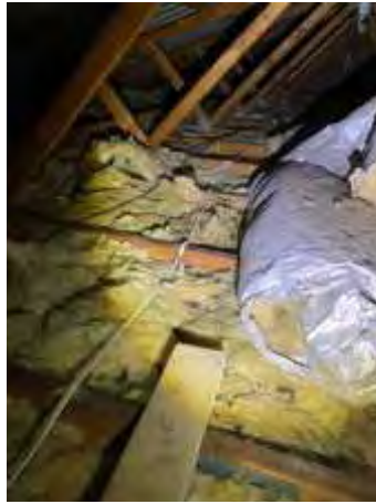
Showing example of metal backed insulation to the roof space
