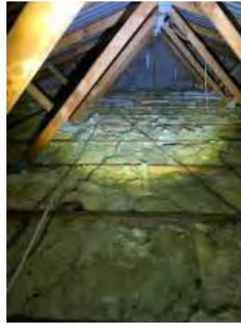
Parts of roof space due to the obstruction
