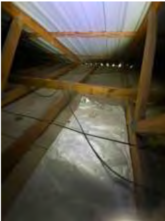
Missing to parts of insulation. Insulation not works as expected. Engaging an insulation technician to refit the missed insulation.
