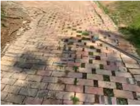
Uneven pathway/driveway, rectify to reduce the risk of people tripping over and personal injury
