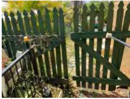
Wood rot to parts of the fences. Recommend engaging a fencing contractor to repair/replace the damaged parts and avoid further deterioration. Make sure all the exposed timbers are painted to maximise the life of the timbers
