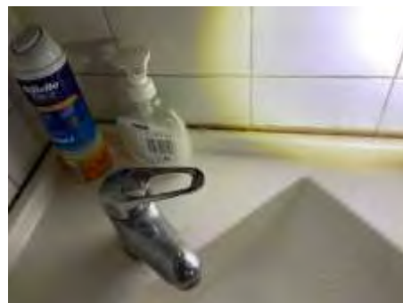
Cracked/loose/missing sealant/grout to parts of bathroom. Recommend resealing to reduce the risk of water leaks and damage
