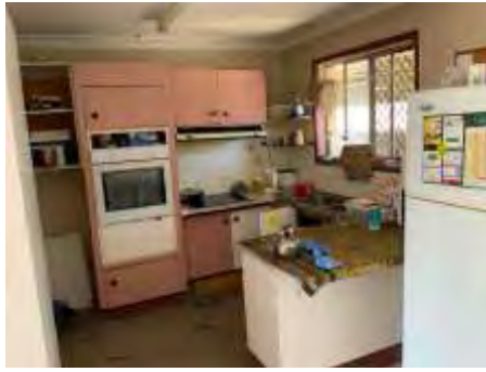
Poor ventilation in Kitchen area. Mould to the ceiling. Needs ventilation improvement
