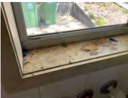
Wood rot to the windows frame. Needs replacement/repair to avoid further deterioration.
