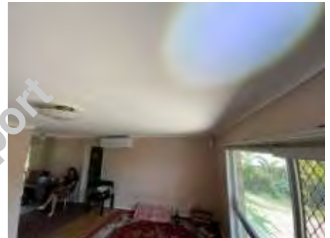
Sagging ceilings. Recommend engaging a plasterer to repair/replace the ceiling to prevent further deterioration,
