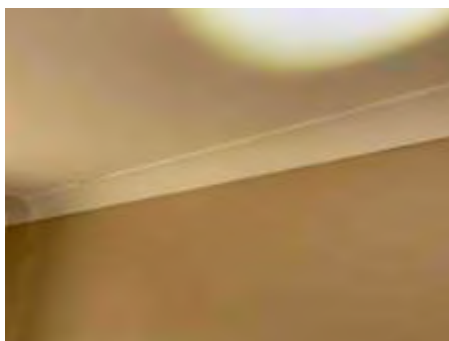
Movement cracks to ceiling and/or cornices. Recommend engaging a plasterer to repairs/replace to prevent further deterioration
