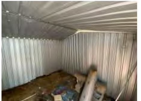
Deterioration to the shed. Needs replacement/repairing
