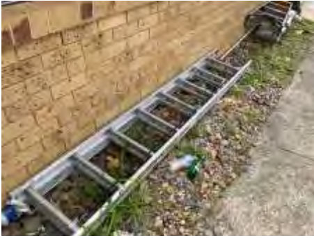
Obstructed weep holes. Recommend exposing 75 mm under the weep holes to reduce the risk of termite attack and water ingress into the building
