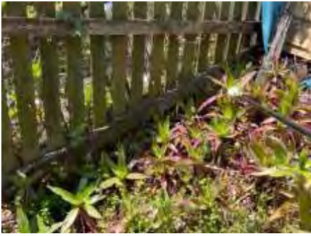
Wood rot to parts of the fences. Recommend engaging a fencing contractor to repair/replace the damaged parts and avoid further deterioration. Make sure all the exposed timbers are painted to maximise the life of the timbers
