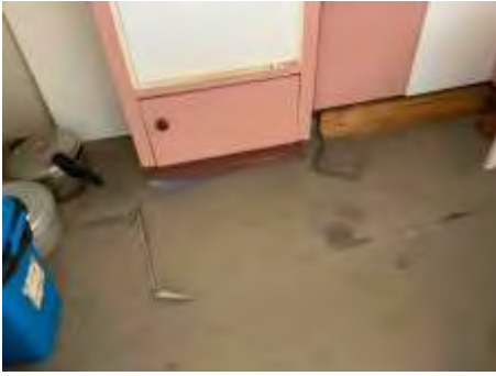
Showing examples of obstructions (e.g. wall, floor, ceiling coverings, cabinets, window furnishings, vegetation, insulation and ducted AC, furniture and stored goods, etc.)
