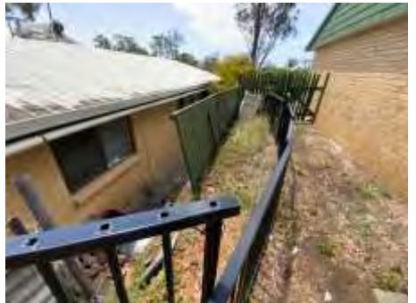
Leaning fences to parts. Recommend engaging a builder/fencer to repair/replace and avoid further deterioration
