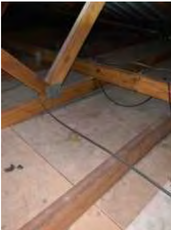
Sagging ceilings. Recommend engaging a plasterer to repair/replace the ceiling to prevent further deterioration,
