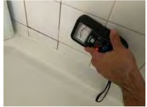
High moisture readings to the walls around the shower. Recommend engaging a builder/plumber for further inspection to determine if the shower needs re-building/waterproofing or it can be repaired easily
