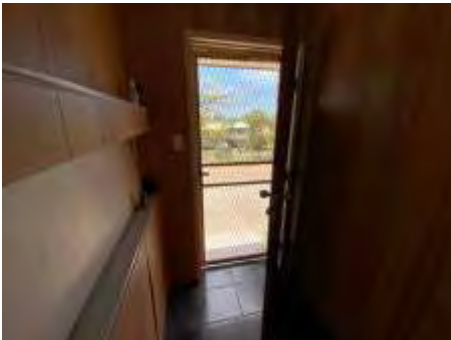
Door is aged/deteriorated. Recommend engaging a carpenter to repair/replace to avoid further deterioration
