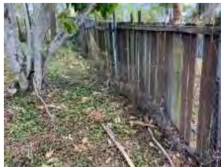
Showing example of bridging/breaching
