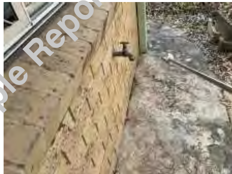
Showing possible source of excessive moisture
