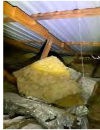
Showing example of metal backed insulation to the roof space
