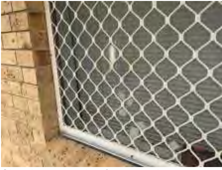
Showing example of torn mesh screen
