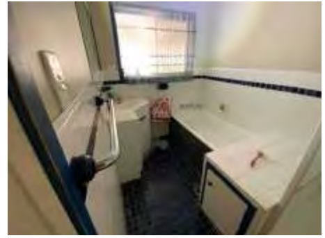
Cracked/loose/missing sealant/grout to parts of bathroom. Recommend resealing to reduce the risk of water leaks and damage
