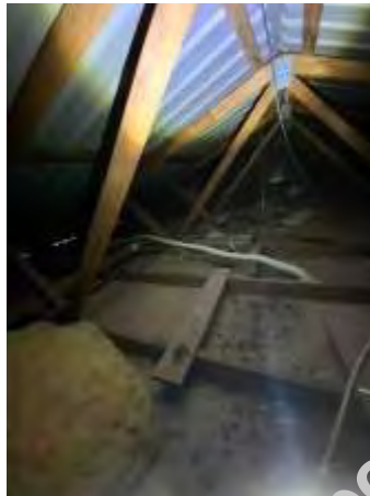
Missing to parts of insulation. Insulation not works as expected. Engaging an insulation technician to refit the missed insulation.
