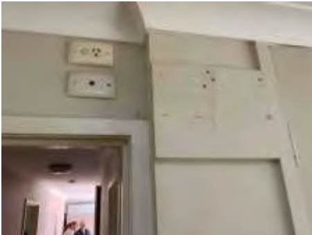
Showing example of scuff marks and paint blemishes
