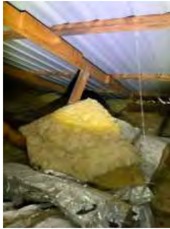
Metal backed insulation installed to the roof space, recommend engaging an electrician and builder to replace the insulation to reduce the risk of electrocution
