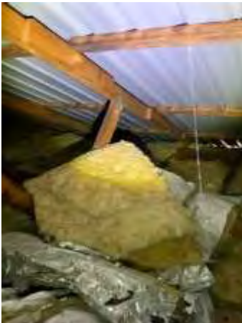
Missing to parts of insulation. Insulation not works as expected. Engaging an insulation technician to refit the missed insulation.
