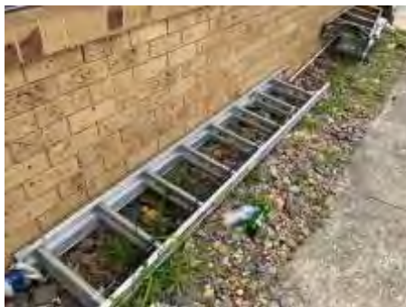
Showing example of bridging/breaching
