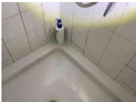
Cracked/loose/missing sealant/grout to parts of bathroom. Recommend resealing to reduce the risk of water leaks and damage
