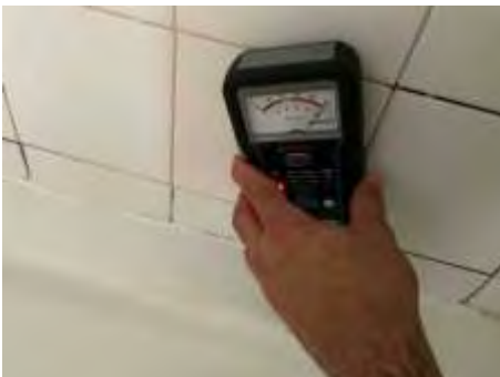
High moisture readings to the walls around the shower. Recommend engaging a builder/plumber for further inspection to determine if the shower needs re-building/waterproofing or it can be repaired easily
