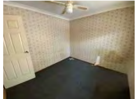
Showing example of scuff marks and paint blemishes
