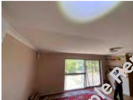
Sagging ceilings. Recommend engaging a plasterer to repair/replace the ceiling to prevent further deterioration,
