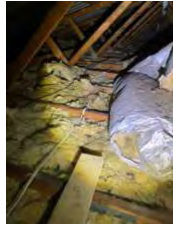
Missing to parts of insulation. Insulation not works as expected. Engaging an insulation technician to refit the missed insulation.
