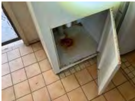
Rust to the laundry cabinet. Replacement needed.
