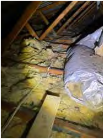
Metal backed insulation installed to the roof space, recommend engaging an electrician and builder to replace the insulation to reduce the risk of electrocution
