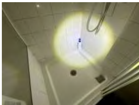
Cracked/loose/missing sealant/grout to parts of bathroom. Recommend resealing to reduce the risk of water leaks and damage
