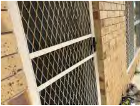
Showing example of minor rusting
