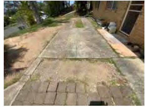
Uneven pathway/driveway, rectify to reduce the risk of people tripping over and personal injury
