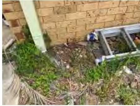
Obstructed weep holes. Recommend exposing 75 mm under the weep holes to reduce the risk of termite attack and water ingress into the building
