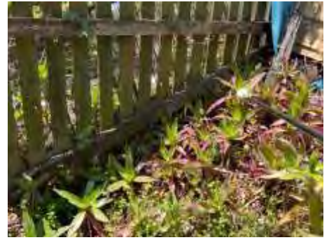
Parts of the fences are in ground contact. Recommend exposing 75mm under the timbers to reduce the risk of wood rot and termite attacks
