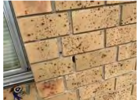
Showing example of missed grout to the external wall
