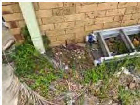
Showing example of bridging/breaching
