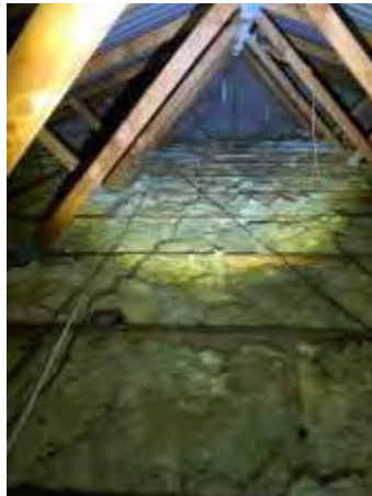
Showing examples of obstructions (e.g. wall, floor, ceiling coverings, cabinets, window furnishings, vegetation, insulation and ducted AC, furniture and stored goods, etc.)
