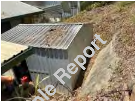
Deterioration to the shed. Needs replacement/repairing
