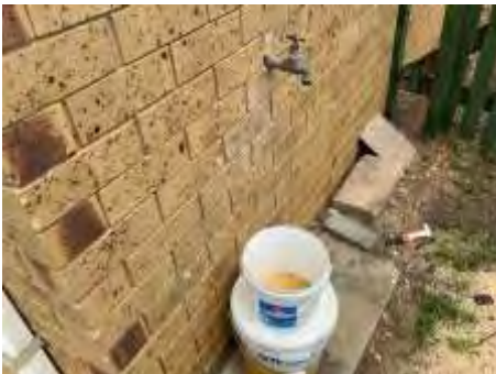
Showing possible source of excessive moisture
