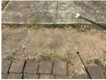
Uneven pathway/driveway, rectify to reduce the risk of people tripping over and personal injury
