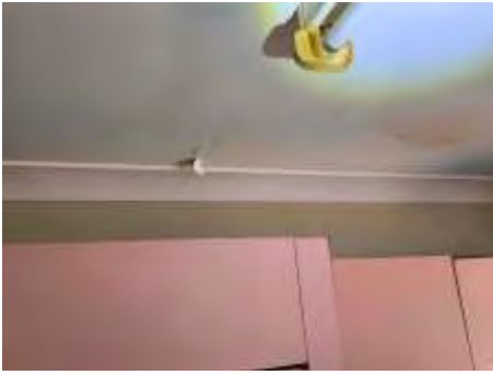
Poor ventilation in Kitchen area. Mould to the ceiling. Needs ventilation improvement
