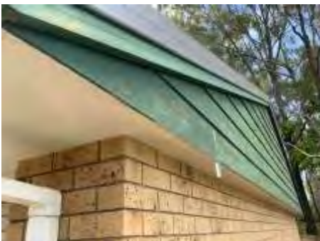
Make sure all the exposed timbers are painted to maximise the life of the timbers
