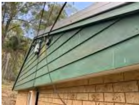
Make sure all the exposed timbers are painted to maximise the life of the timbers
