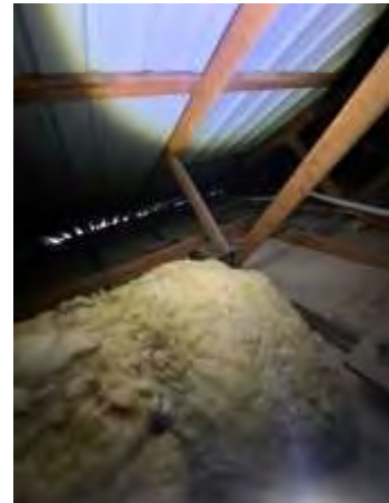
Missing to parts of insulation. Insulation not works as expected. Engaging an insulation technician to refit the missed insulation.
