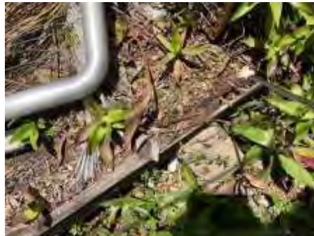
Wood rot to parts of the retaining walls. Recommend engaging a builder to repair/replace and avoid further deterioration
