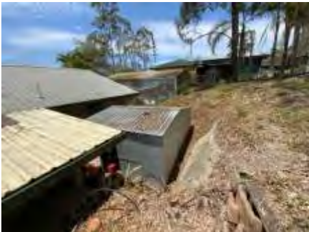
Deterioration to the shed. Needs replacement/repairing
