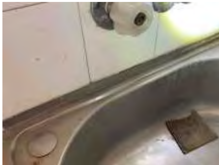
Joins to Laundry tub splash back needs resealing to reduce the risk of water leaks and penetration,
