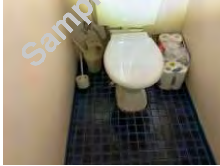
Cracked/loose/missing sealant/grout to parts of bathroom. Recommend resealing to reduce the risk of water leaks and damage
