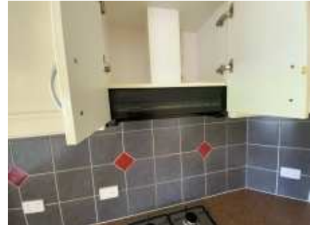
Showing the broken range hood, an electrician recommended to repair/replace and make it usable
