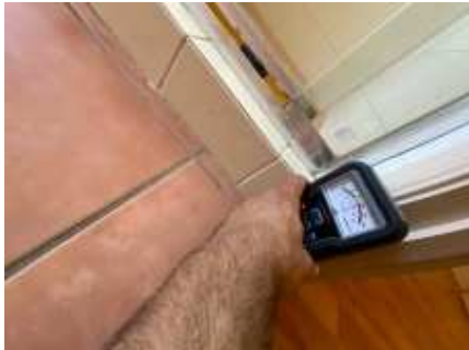
Showing possible source of excessive moisture
