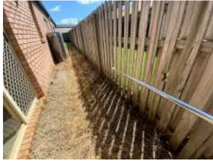
Showing example of the bridging/breaching
