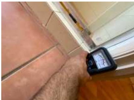
High moisture readings to the walls around the shower. Recommend engaging a builder/plumber for further inspection to determine if the shower needs re-building/waterproofing or it can be repaired easily, Behind the main bathroom shower wall, to the floor and door frame
