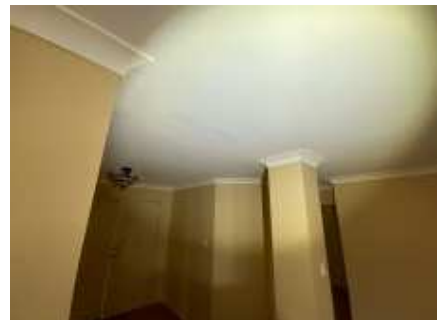
Movement cracks to ceiling and/or cornices. Recommend engaging a plasterer to repairs/replace to prevent further deterioration, Living room
