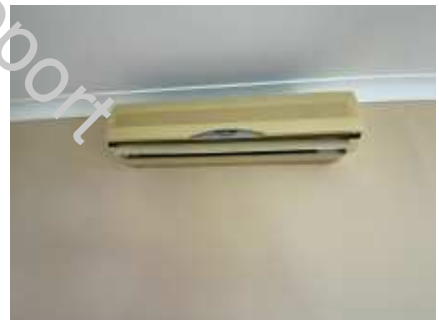
Air conditioning panel remained open, after turning off, an electrician recommended
