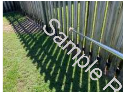
Parts of the fences are in ground contact. Recommend exposing 75mm under the timbers to reduce the risk of wood rot and termite attacks
