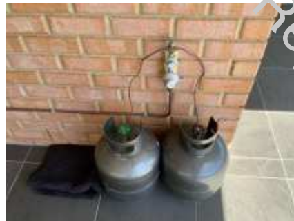
It appears the bottles gas are empty., Any services requiring gas will be inoperable. Recommend further investigations once gas bottles are connected to ensure correctly installed and all services operating correctly. Recommend the above be implemented as soon as practicable
