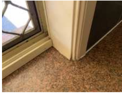
Wood rot/water damage to the kitchen window timber frame, a carpenter recommended to repair/replace and avoid further deterioration
