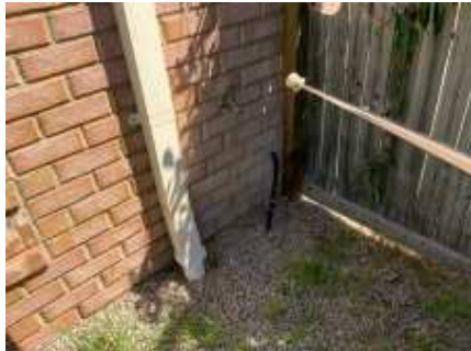
Showing possible source of excessive moisture
