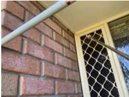
Showing example of settlement cracks, Soffit sheet moulding
