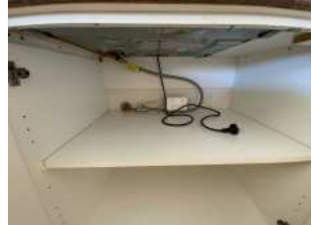
The power point under cook top is not working, an electrician recommended
