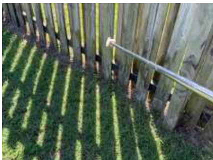
Wood rot to parts of the fences. Recommend engaging a fencing contractor to repair/replace the damaged parts and avoid further deterioration. Make sure all the exposed timbers are painted to maximise the life of the timbers
