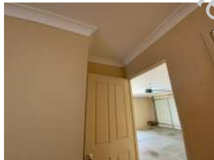
Showing sagging to the ceiling, top of the garage door
