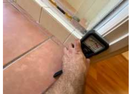
High moisture readings to the walls around the shower. Recommend engaging a builder/plumber for further inspection to determine if the shower needs re-building/waterproofing or it can be repaired easily, Behind the main bathroom shower wall, to the floor and door frame
