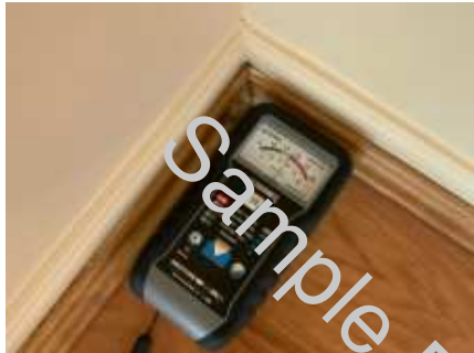
Showing possible source of excessive moisture
