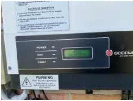
Showing solar panel is working at the time of the inspection, but an electrician recommended to inspect the energy efficiency of the solar units
