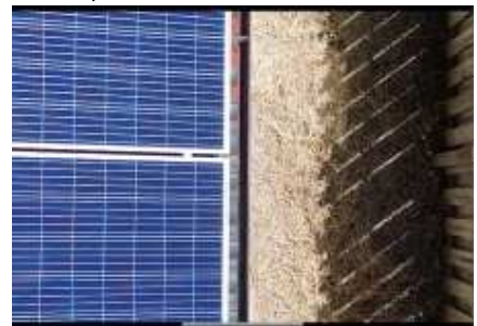
Showing minor scratches to the solar panel
