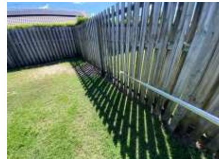
Wood rot to parts of the fences. Recommend engaging a fencing contractor to repair/replace the damaged parts and avoid further deterioration. Make sure all the exposed timbers are painted to maximise the life of the timbers
