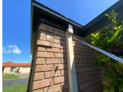
Water stain on front downpipe, it looks like is leaking, a plumber recommended
