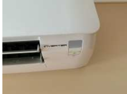
All AC units were working at the time of the inspection, but for a proper testing and gas measurement, a AC technician needs to be engaged
