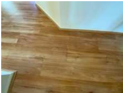
Showing example of the damaged floor board
