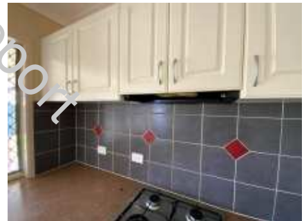
The rangehood is broken, an electrician recommended.
