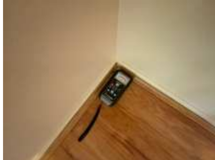
High moisture readings to the walls around the shower. Recommend engaging a builder/plumber for further inspection to determine if the shower needs re-building/waterproofing or it can be repaired easily, Behind the main bathroom shower wall, to the floor and door frame
