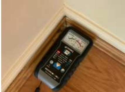
High moisture readings to the walls around the shower. Recommend engaging a builder/plumber for further inspection to determine if the shower needs re-building/waterproofing or it can be repaired easily, Behind the main bathroom shower wall, to the floor and door frame
