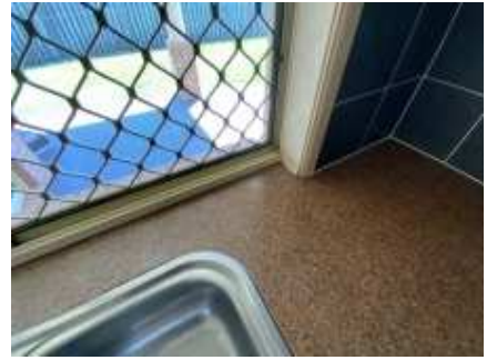
Wood rot/water damage to the kitchen window timber frame, a carpenter recommended to repair/replace and avoid further deterioration
