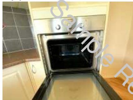
Oven was working at the time of the inspection, but an electrician recommended to test the oven energy efficiency., Some written guides around the knobs are unreadable
