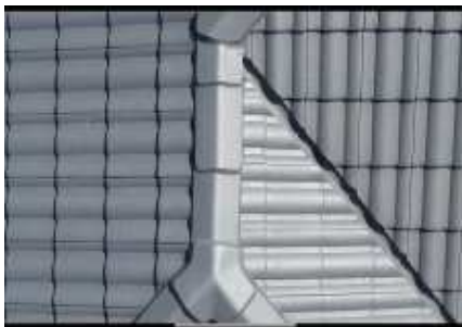
Showing example of settlement cracks, Roof tile, minor scratches.
