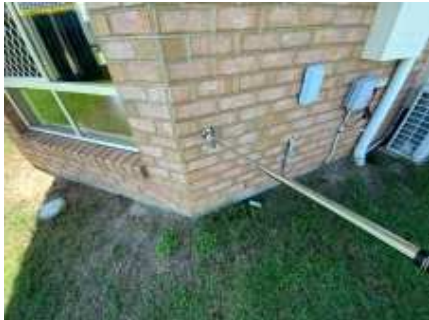
Showing possible source of excessive moisture
