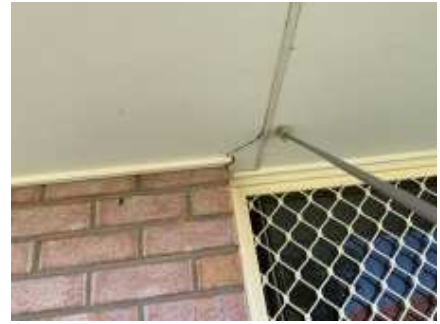
Showing example of the damaged soffit sheet
