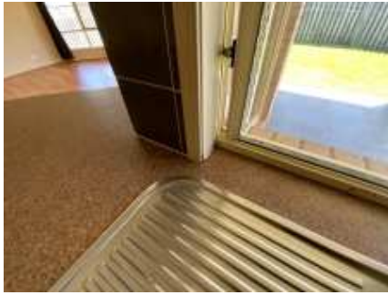
Wood rot/water damage to the kitchen window timber frame, a carpenter recommended to repair/replace and avoid further deterioration
