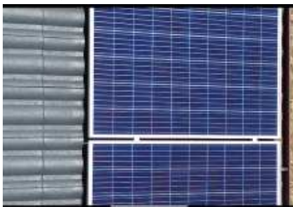
Showing minor scratches to the solar panel
