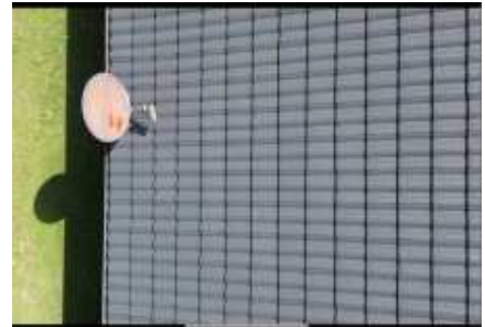
Showing example of minor rusting
