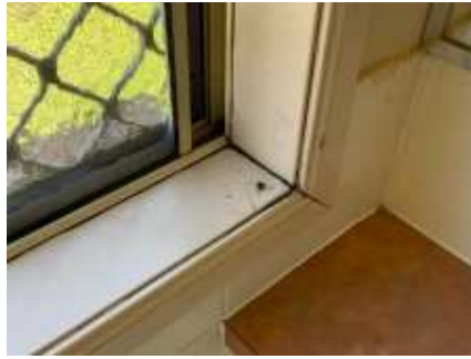
Moisture damage to the windows frame, recommend engaging a carpenter to repair/replace the affected area and avoid further deterioration
