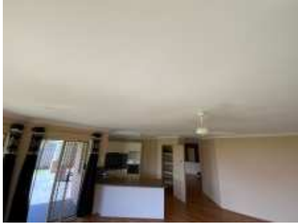
Sagging ceilings. Recommend engaging a plasterer to repair/replace the ceiling to prevent further deterioration,, Dining room
