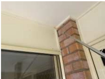
Showing example of the minor gap around door/windows frame, recommend applying silicone to avoid water entry to the wall
