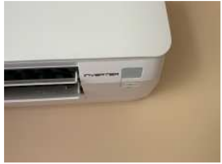
All AC units were working at the time of the inspection, but for a proper testing and gas measurement, a AC technician needs to be engaged
