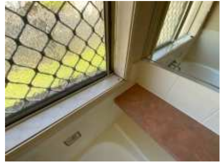
Moisture damage to the windows frame, recommend engaging a carpenter to repair/replace the affected area and avoid further deterioration
