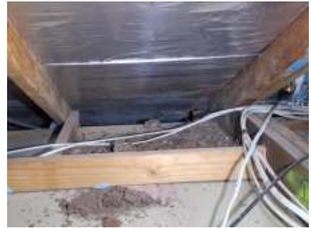
Showing sign of the termite working inside the roof space
