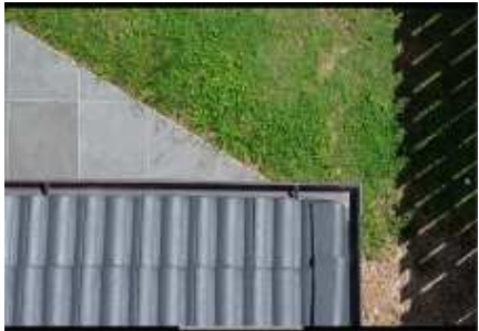
Showing possible source of excessive moisture
