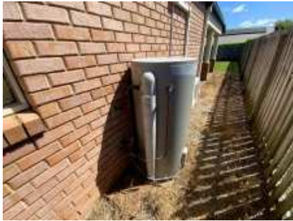
Showing example of the bridging/breaching
