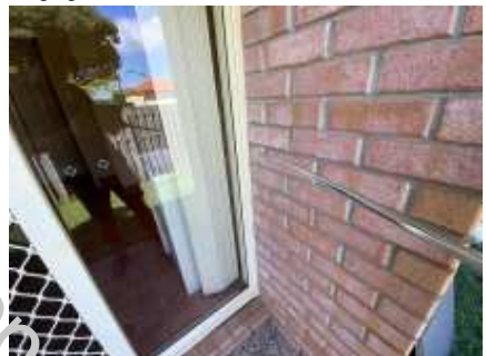
Showing example of the minor gap around door/windows frame, recommend applying silicone to avoid water entry to the wall
