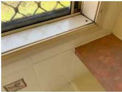
A few cracked tiles to the bathroom. Recommend engaging a tiler to repair/replacing to reduce the risk of water leaks and damage, Movement crack to the wall which affected the tile's mortars
