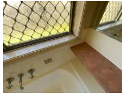
A few cracked tiles to the bathroom. Recommend engaging a tiler to repair/replacing to reduce the risk of water leaks and damage, Movement crack to the wall which affected the tile's mortars
