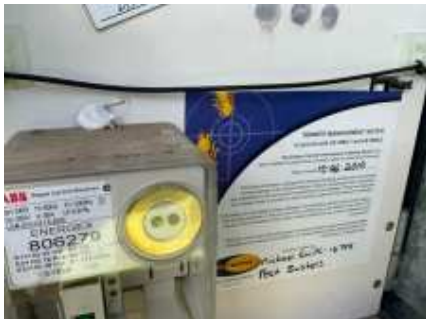
Showing sign of termite management system in meter box.
