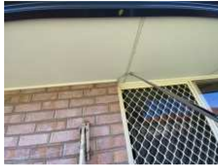
Showing example of the damaged soffit sheet
