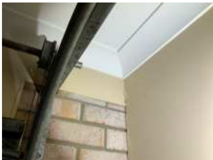
Showing example of settlement cracks, Wall/cornices
