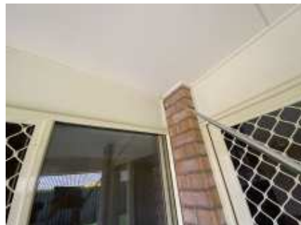
Showing example of the minor gap around door/windows frame, recommend applying silicone to avoid water entry to the wall
