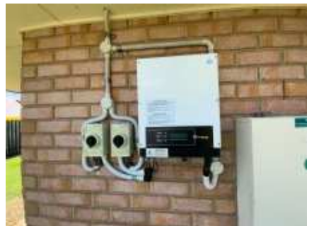
Showing solar panel is working at the time of the inspection, but an electrician recommended to inspect the energy efficiency of the solar units
