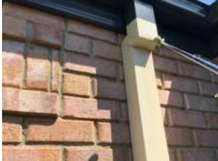
Water stain on front downpipe, it looks like is leaking, a plumber recommended
