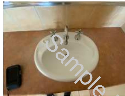
Cracked/loose/missing sealant/grout to parts of bathroom. Recommend resealing to reduce the risk of water leaks and damage
