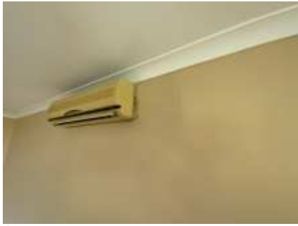
Showing example of the previous attempt to repair the wall
