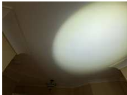
Movement cracks to ceiling and/or cornices. Recommend engaging a plasterer to repairs/replace to prevent further deterioration, Living room
