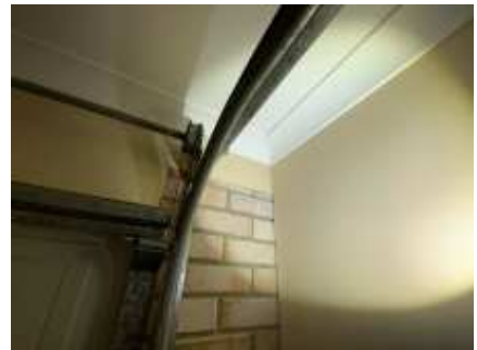
Showing example of settlement cracks, Wall/cornices
