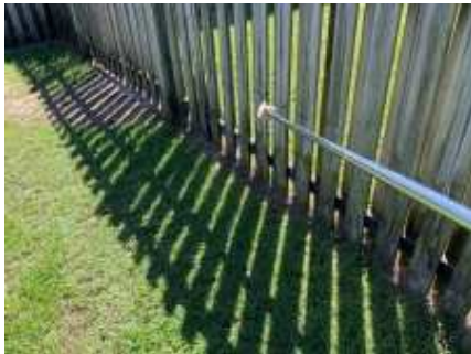
Showing example of the wood rot to the timber
