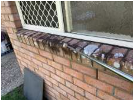
Showing example of the mould/moisture stain to the wall
