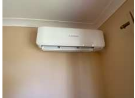
All AC units were working at the time of the inspection, but for a proper testing and gas measurement, a AC technician needs to be engaged
