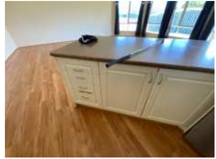
Showing example of loose/missing laminate to the cabinets
