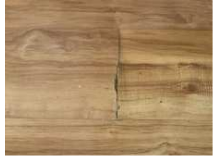
Showing example of the damaged floor board
