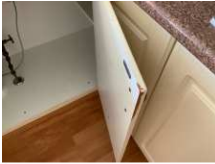
Showing example of loose/missing laminate to the cabinets
