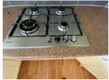
Any services requiring gas will be inoperable when the gas bottles are empty. Recommend further investigations once gas bottles are connected to ensure correctly installed and all services operating correctly. Recommend the above be implemented as soon as practicable. It looks no electricity is connected to the cabinet powerpoint, under cook top.
