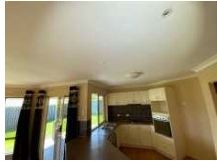
Sagging ceilings. Recommend engaging a plasterer to repair/replace the ceiling to prevent further deterioration,, Dining room
