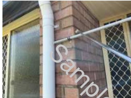
Showing example of minor rusting
