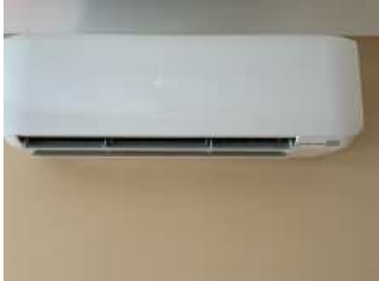
All AC units were working at the time of the inspection, but for a proper testing and gas measurement, a AC technician needs to be engaged
