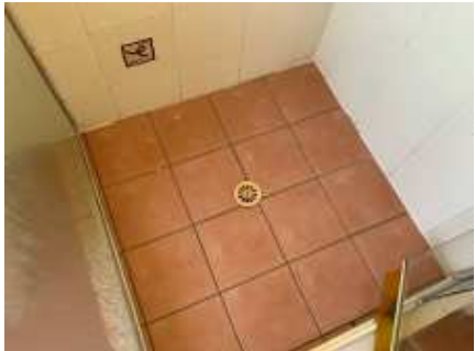
Showing possible source of excessive moisture
