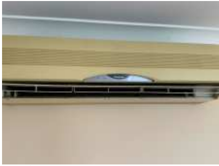
All AC units were working at the time of the inspection, but for a proper testing and gas measurement, a AC technician needs to be engaged
