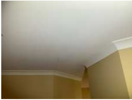
Movement cracks to ceiling and/or cornices. Recommend engaging a plasterer to repairs/replace to prevent further deterioration, Living room
