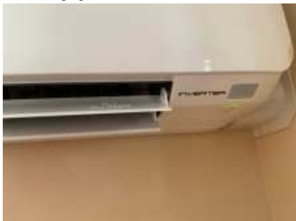
All AC units were working at the time of the inspection, but for a proper testing and gas measurement, a AC technician needs to be engaged
