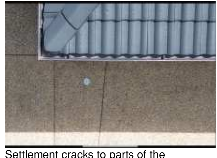
Settlement cracks to parts of the pathway/driveway. Recommend engaging a concreting contractor to repair/replace and avoid further deterioration
