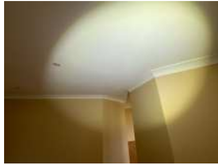
Movement cracks to ceiling and/or cornices. Recommend engaging a plasterer to repairs/replace to prevent further deterioration, Living room
