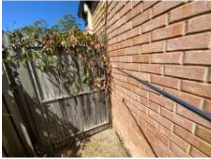
Showing example of the bridging/breaching
